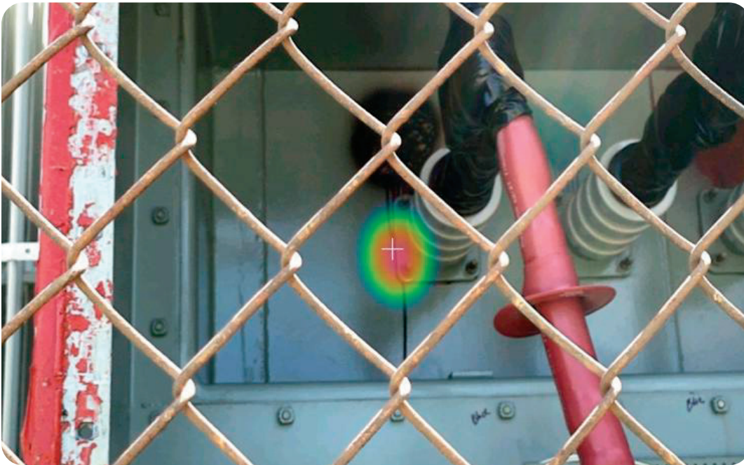
Si2-PRO Acoustic Camera identification of the sound source at the transformer bushing connection.
